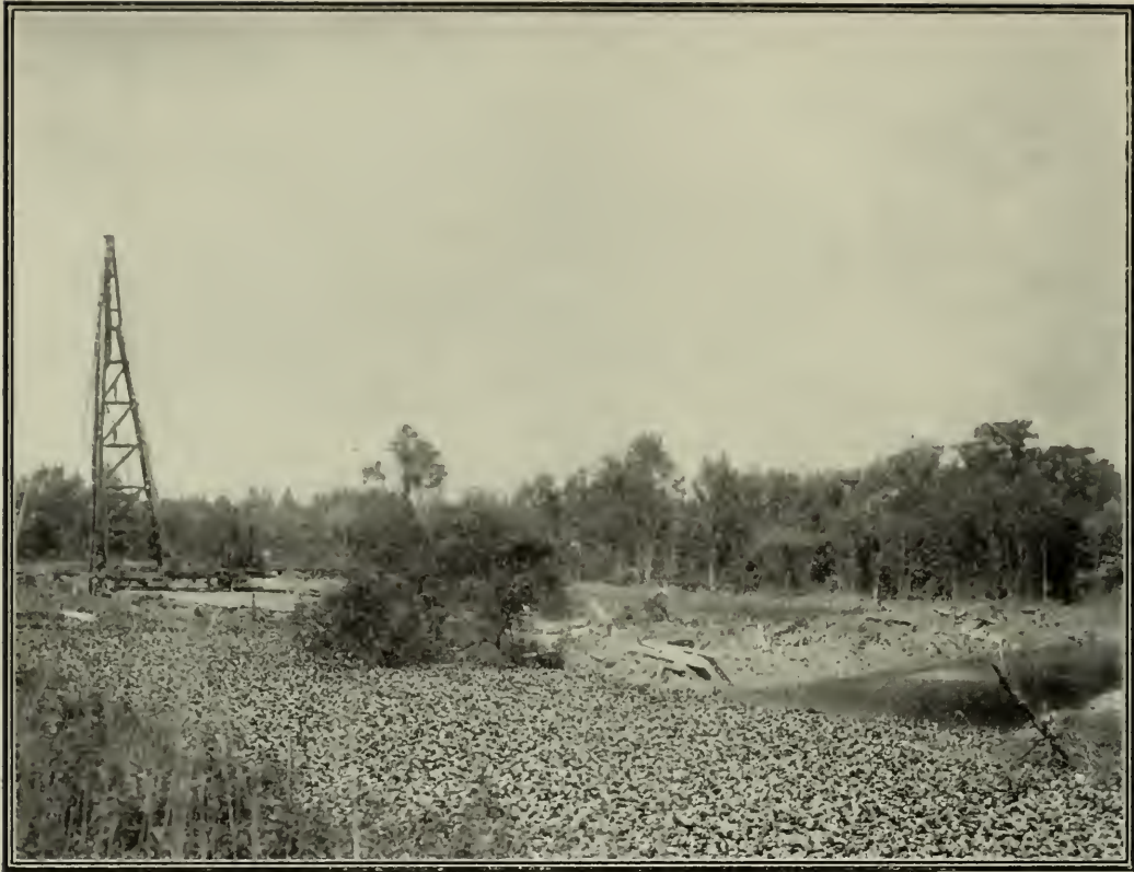
SITE OF PUMPING STATION NO. 6, SHOWING BY-PASS, PILE DRIVER, AND OLD CANAL FILLED WITH WATER HYACINTHS.
